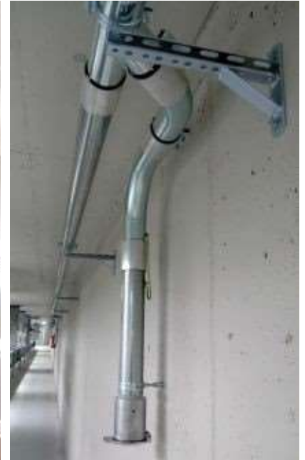
Metal central vacuum cleaner pipeline
