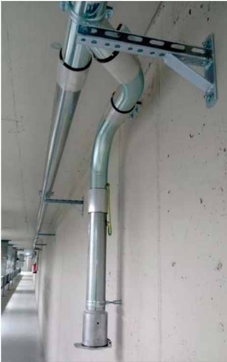
Central suction pipe
