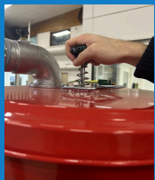
Manual filter cleaning
