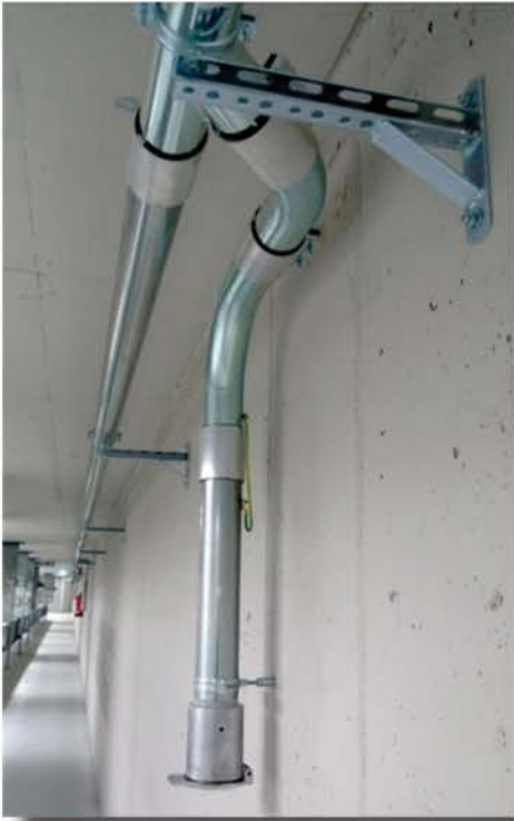
Central suction pipe
